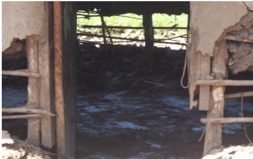
Plate.1: House Destroyed by Floods
